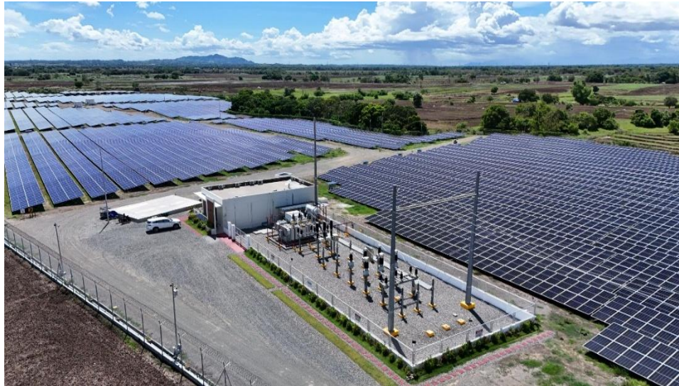
The SJSP uses 24,675 units of 670Wp and 4,564 units of 675Wp PV panels supplied by Trina Solar and 51 units of 300kVA Huawei string inverters.
